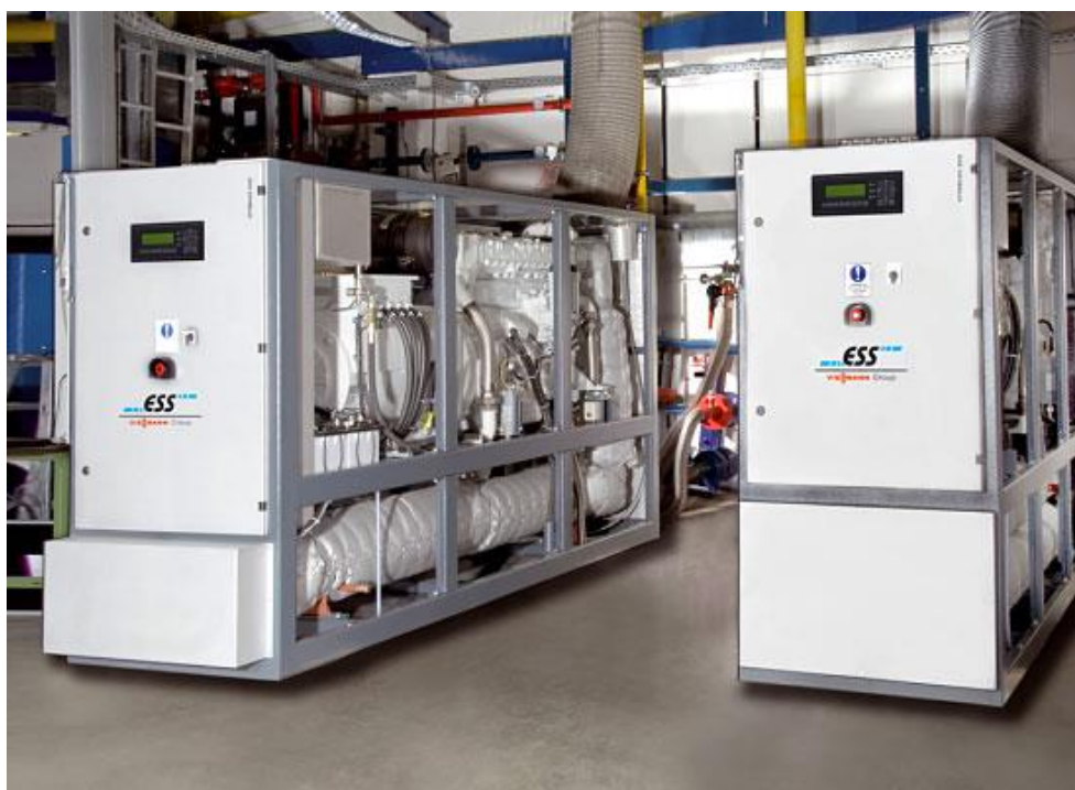
400kW Natural Gas CHP Plant. Photo Courtesy of www.viessmann.co.uk
